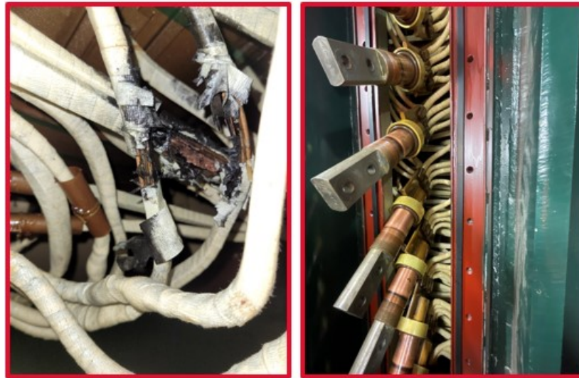
Figure 2. Illustration of the type of damage found in the rectifiers due to overheating.
